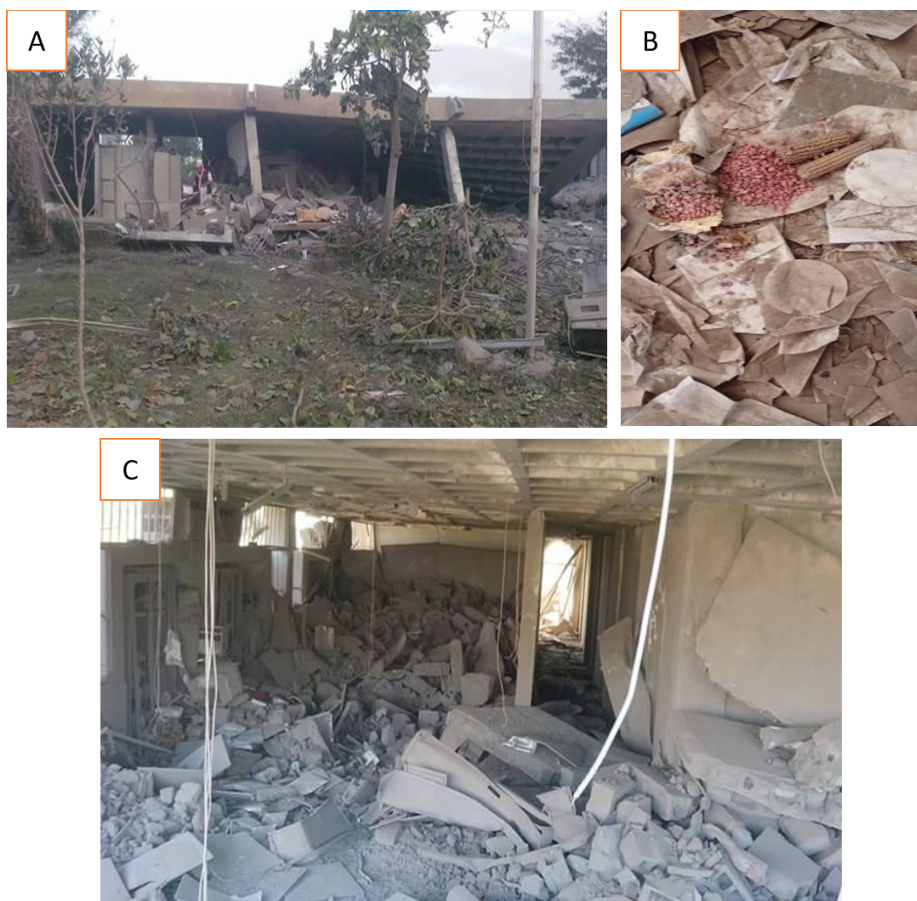
Figure 1. Examples of the effects of the air raids of the war coalition against Yemen on the buildings, equipment and seed stores of the Tehama regional agricultural research station in the western coastal plain, Al-Kadan, Sardoud, Tihama zone, Al-Hodeidah governorate (A and C), including damage to the preserved seed samples of various crops (B).
